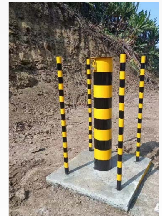
Groundwater Monitoring Well
